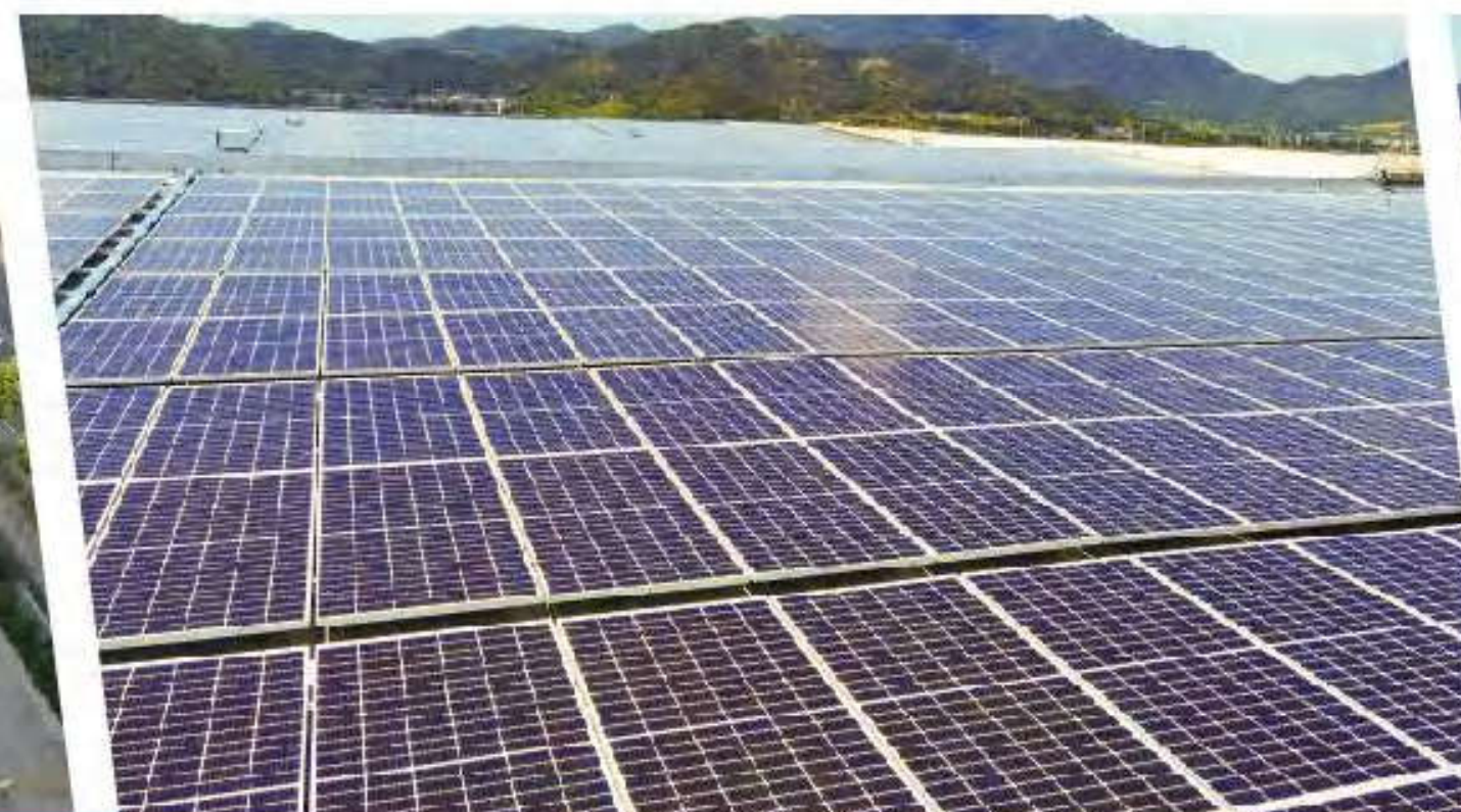
▶ Ningbo Xiangshan 5.7 MWp Project
