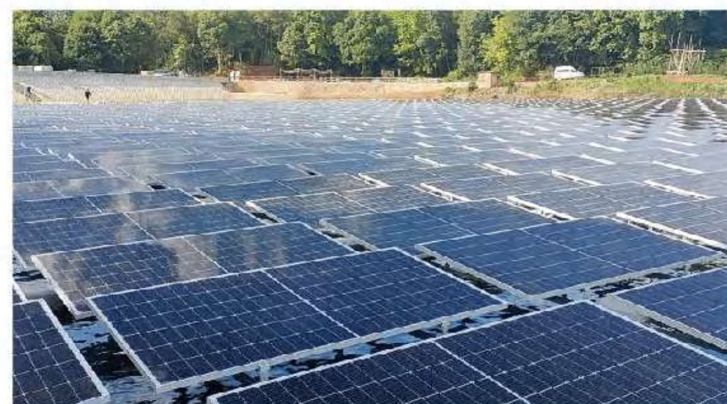
▶ Shaoxing 2MWp Surface Power Station
